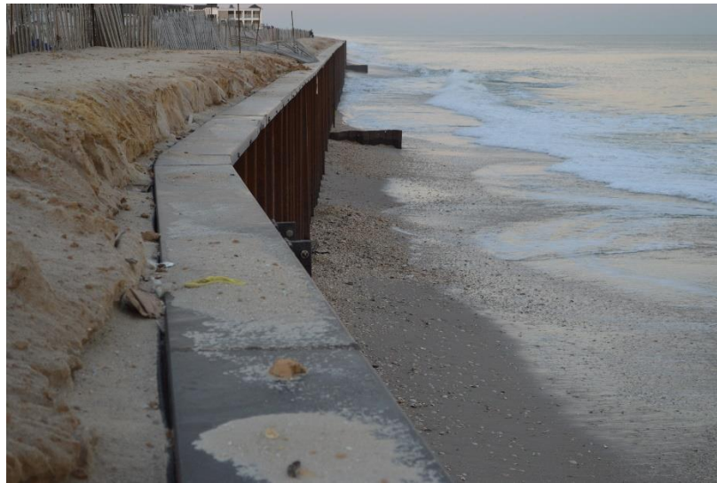
Figure 11. Erosion toward face of sea wall.
