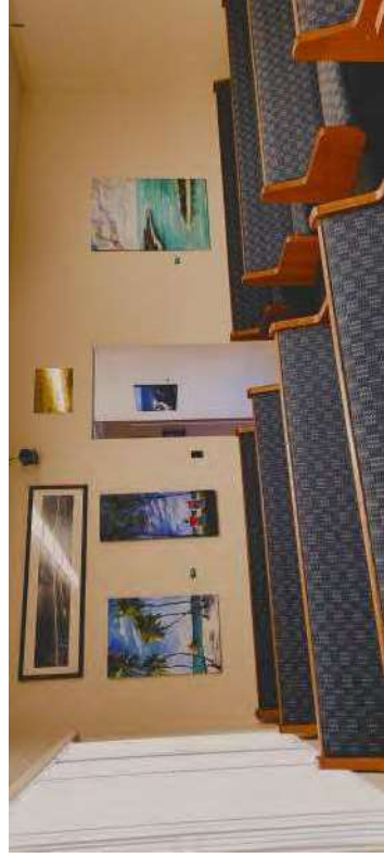
Existing seating pews in chamber (ADA Non Compliant)
