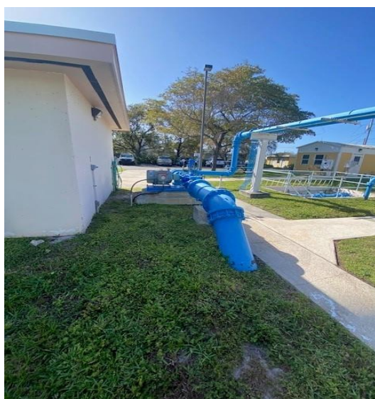
WTP HS Pump
