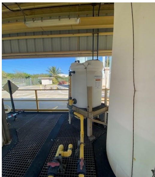
Chlorine Bulk & Day Tank
