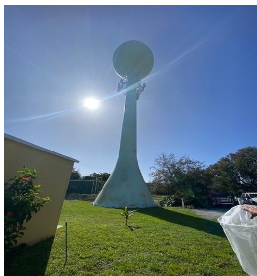
Disconnected Elevated Tank
