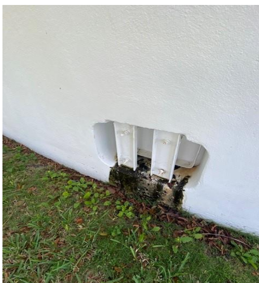
Leaking GST Entry Point
