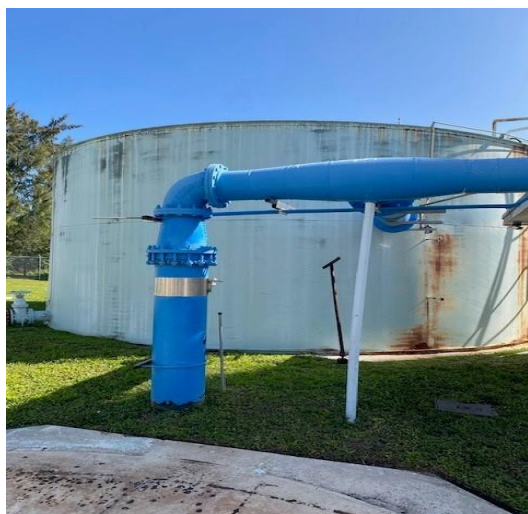
Clearwell (To be Replaced)
